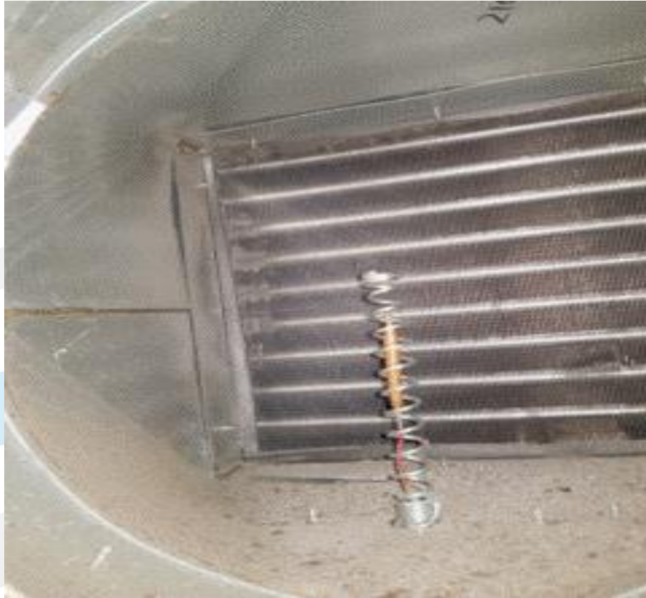
Heavily contaminated and blocked heating coil
