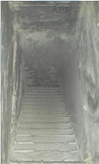
Supply duct before cleaning
