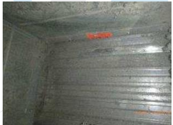
Heavily regulated damper blocked
