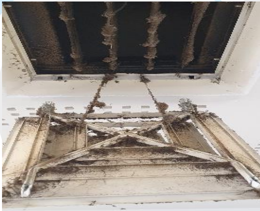
Heavy Contamination on grille and damper.
